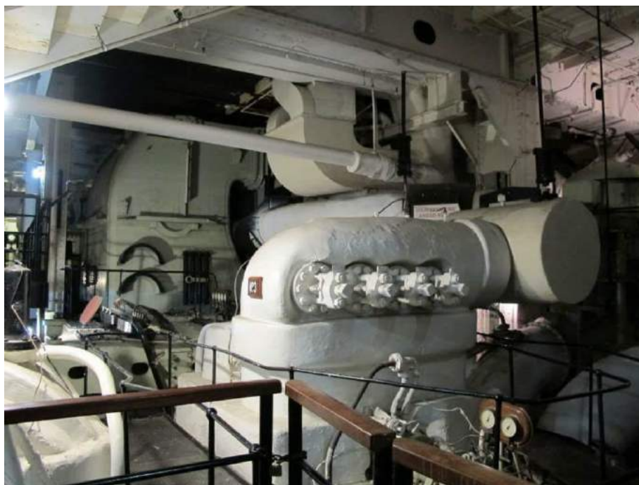
Figure 43 - Starboard after nozzle bank today - on top of HP turbine
