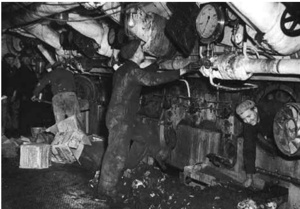
Figure 69 - a propulsion boiler in Boiler Room 2 undergoing maintenance
