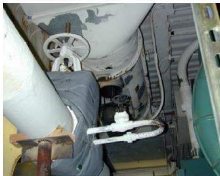
Figure 38 – warming through line on main valve
